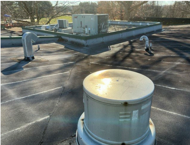
15 - ROOFTOP HVAC EQUIPMENT
